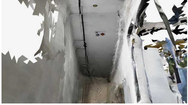
(b) A NIST ring target on the ceiling of an unlit room
